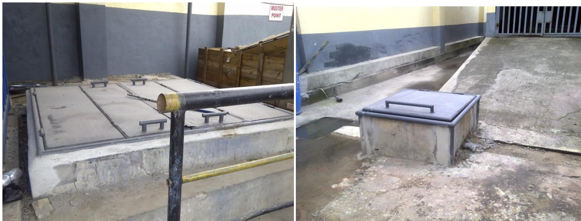
SECONDARY CONTAINMENT TO DISCHARGE EFFLUENT AND TO WASH OFF SPILLS
