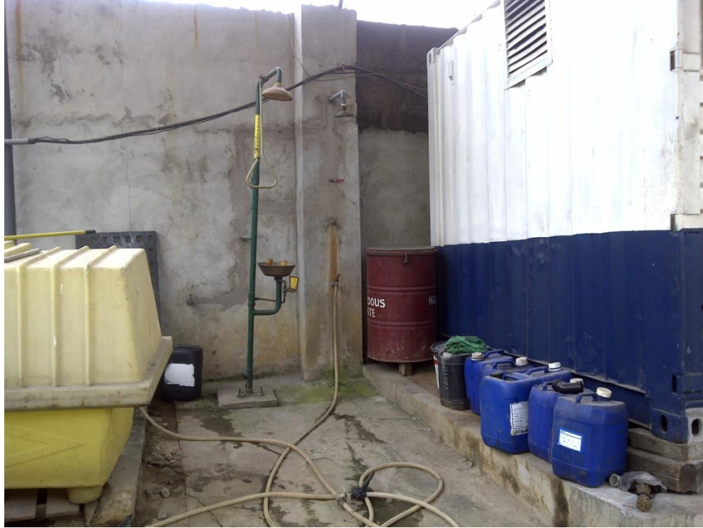
EYE WASH/SHOWER STATION AT THE BULKING AREA
