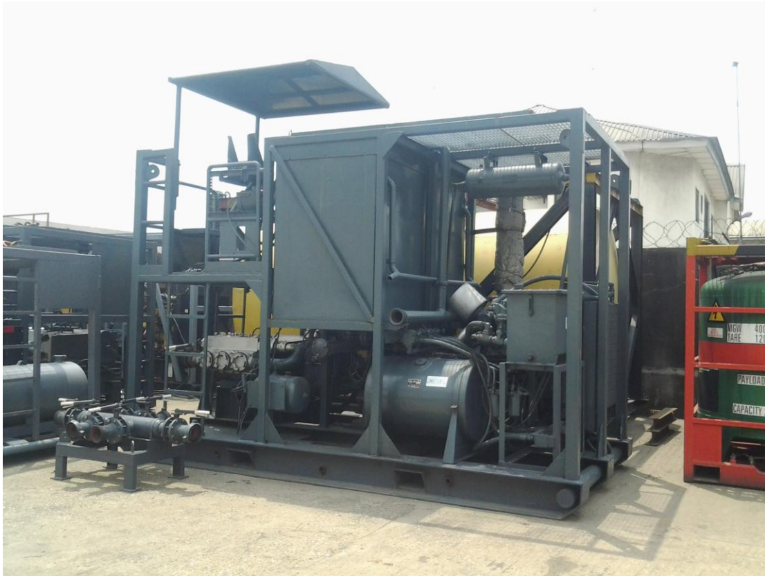
Single pump Unit with Manifold
